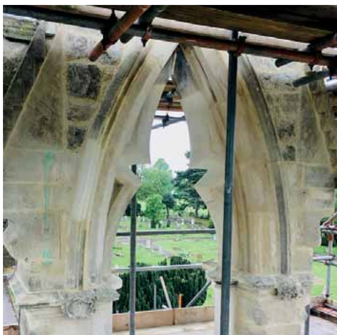
Partially rebuilt Belcote – part of a grade II listed building at the Council's Bell Road Cemetery
